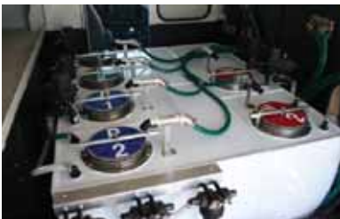
Six Tank System (Single to multiple systems available)
